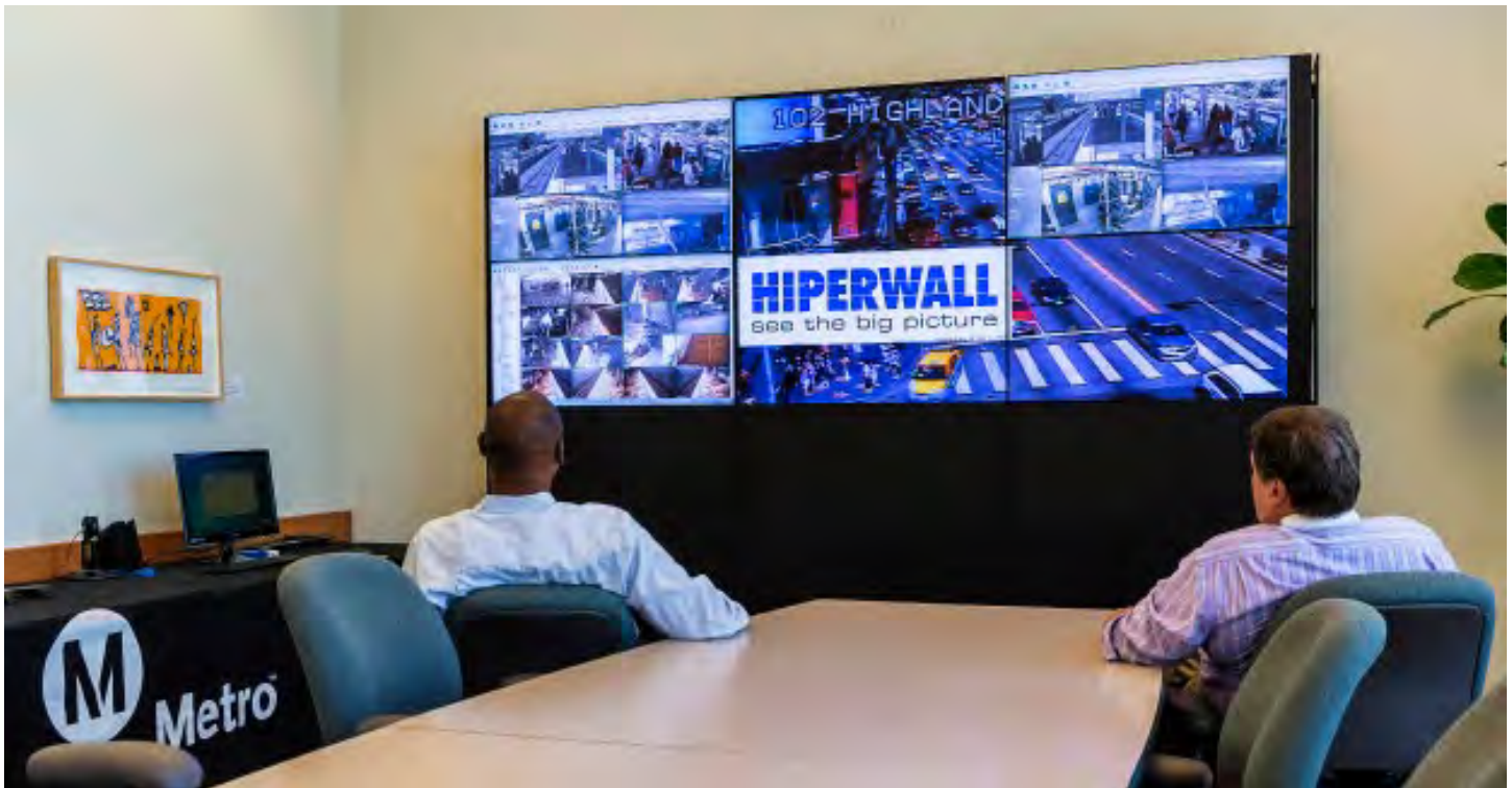
On the sixth floor, LA Metro staff choose which visual intelligence is important for LA Metro executives to see, and then they share only that content on a second wall in the executive briefing room, located on the 26 th floor.
